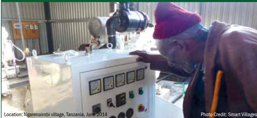
Exhibit B: The village micro-grid is powered by a 300 kW biofuel generator fuelled by locally grown Jatropha
