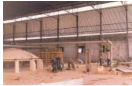
(ii) Recuperator to burner
