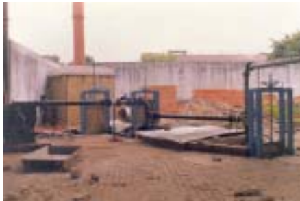
(i) Blower to recuperator
